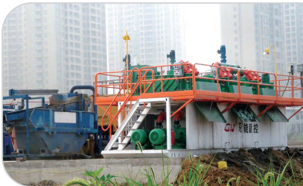
Dredging Slurry Solids and Liquid Separation
