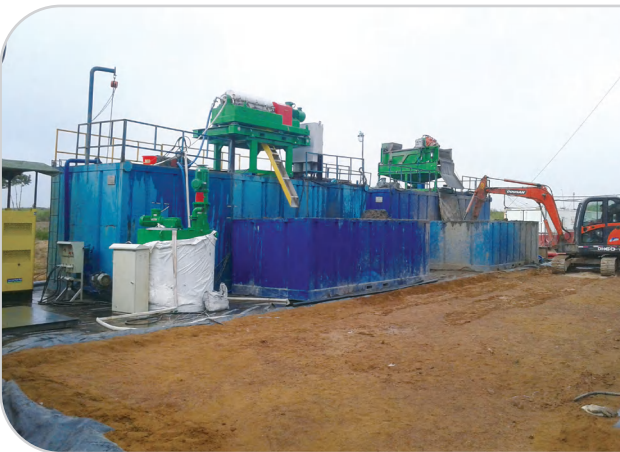
Inner Mongolia WBM Treating Project
